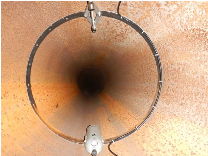
As installed at Big Spring Fish Hatchery
